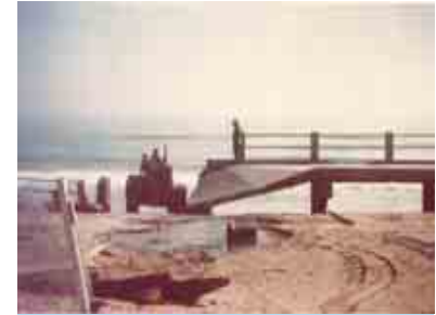
Ash Wednesday damage to Boardwalk
