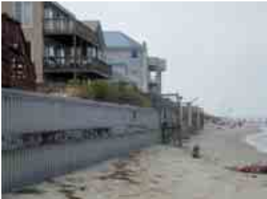
Effects of erosion
