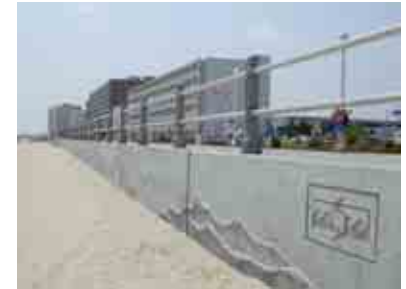
Seawall at the Resort Beach
